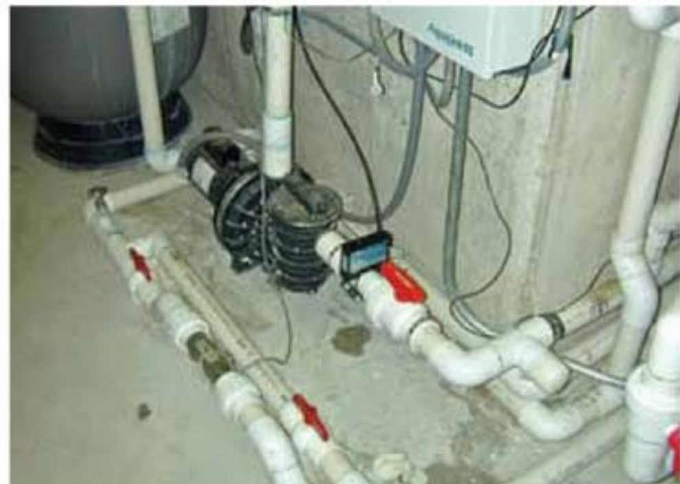
TOPS installed the new conditioning system in an effort to decrease the use of chemicals to control water quality.
