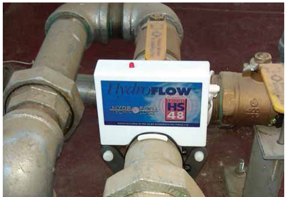
Green-HVAC Solutions installed a model HS-48 conditioner in each of the three Brookfields Restaurants.
