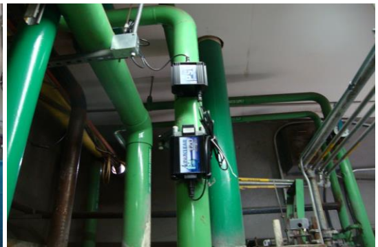
Installed HydroFLOW 120 Water Conditioner
